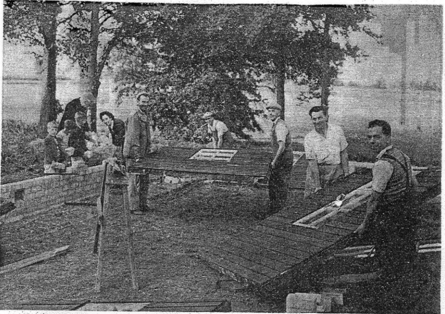
THE BUSY SCENE on Wednesday evening, when the volunteers were hard at work erecting the new Church Hall. Seen in the picture are the Vicar (Rev J. A. Sangster) and Mrs. Sangster, Messrs. Harold Daniels, L. Russell, Jack Bates, Junr., C. Horrey and G. Horrey—not forgetting the young helpers, who have also been doing their full share of fetching and carrying—Roger Cooper, David Watson and Martin Bates.
